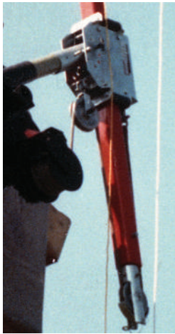
Winch line connects to mast base to raise conductors and provide working clearances for operator.
