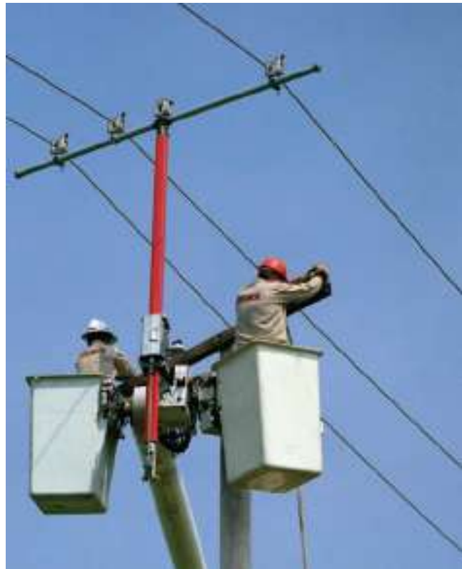
Wireholders latch easily from bucket with hookstick. 12" Epoxirod link insulates each latch-release lanyard.
